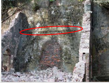
Tie rods in church ruins
